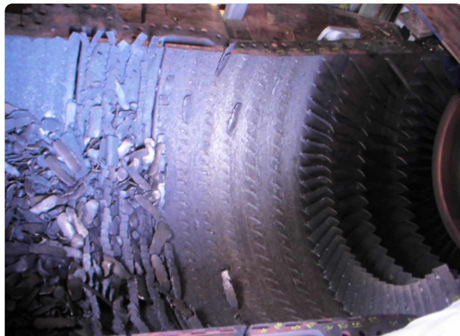
FIGURE 1. Lower compressor casing after large forward blade liberation, causing a forced outage and catastrophic damage to aft components.
