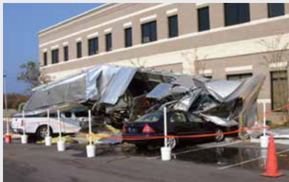
18,000 lb AHU Blown off Roof, Hurricane Katrina, Mississippi (FEMA 2005)
